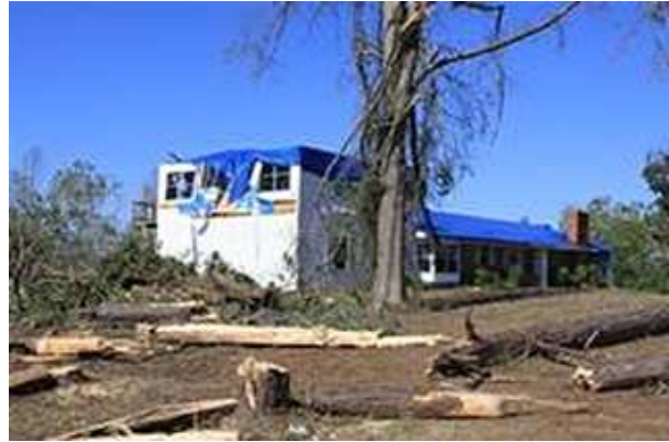
FIG. 7. House with EF2 damage.
