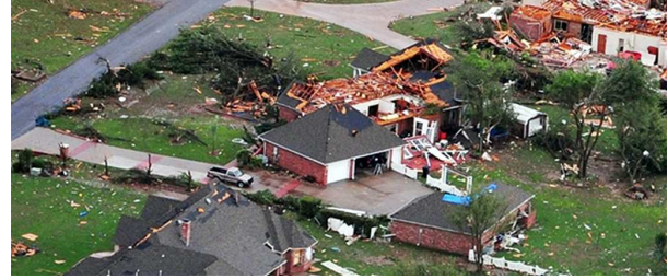
FIG. 11. The same structure shown in Fig. 9 captured from a helicopter. Image source: USA Today.
