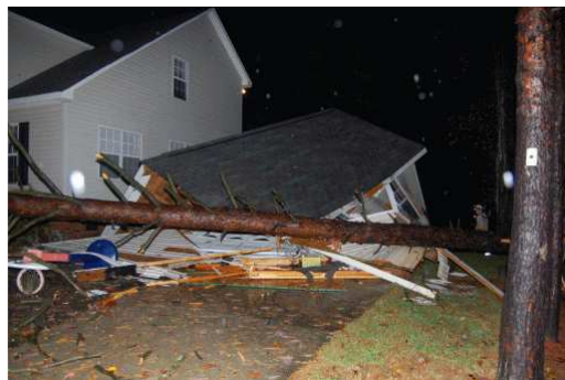
Fig. 6. One of the greatest dangers associated with downbursts in the western Carolinas and northeast Georgia is from falling trees. Every year, falling trees result in millions of dollars in damage to property across the region. Injuries and even fatalities also occur from time to time.
