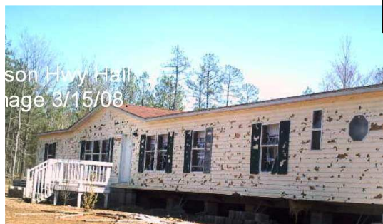
Fig. 7. Damage to a manufactured home by large hail up to the size of baseballs. Large hail is responsible for billions of dollars in property losses across the United States each year. The damage in this photo occurred on March 15, 2008 near Callison, SC. Photo courtesy of Greenwood County Emergency Management.
